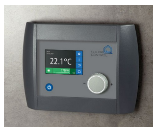
Solar Control Panel
