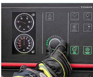
Control element for pump control station
