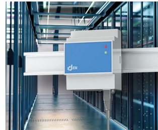
Energy management in data centres
