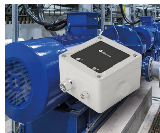
Sensor box for system monitoring
