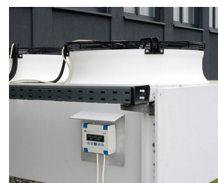
Heating/air conditioning/ventilation control
